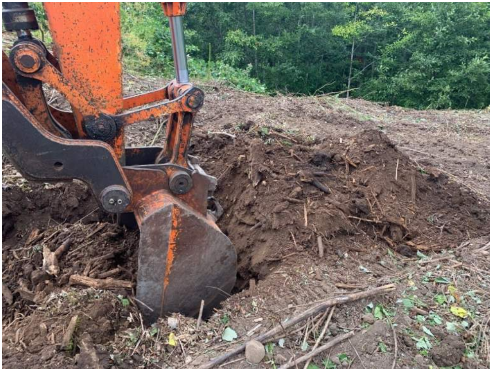
Photo 1: An excavator was used during sampling to ensure that “fresh” samples were obtained for chemical testing to reduce the potential loss of volatile contaminants.
